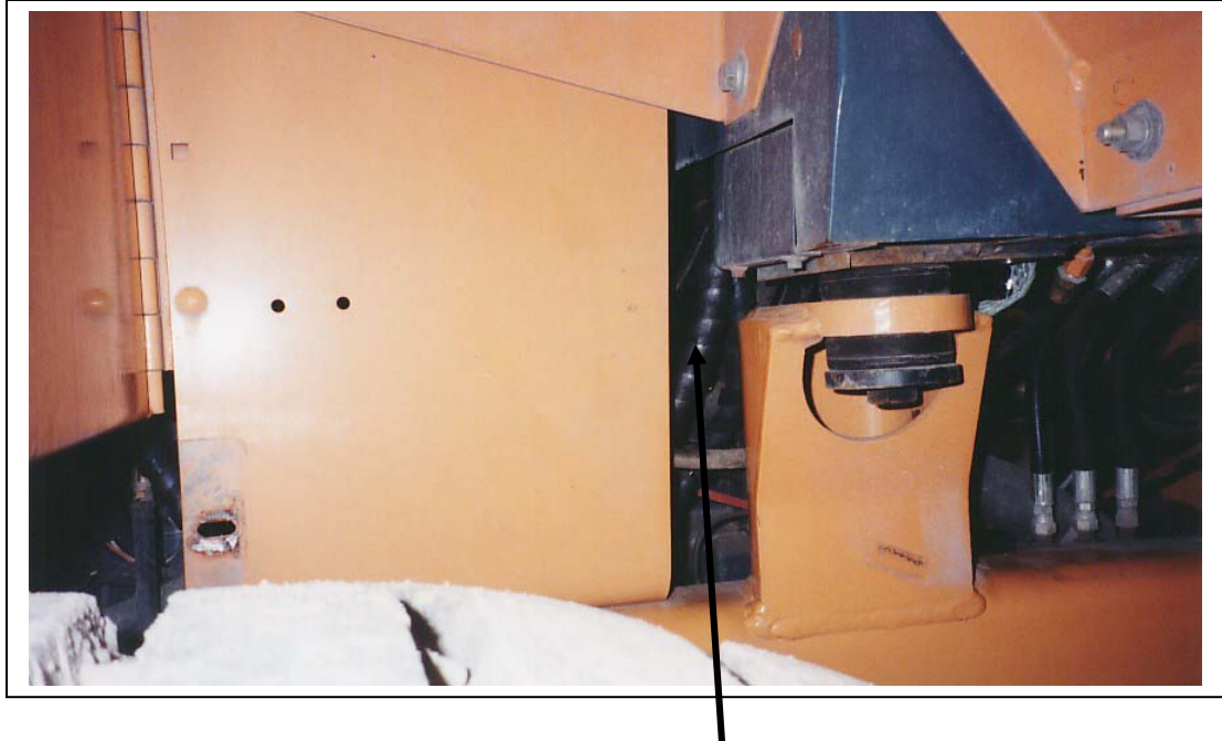
A/C hoses entering the cab
