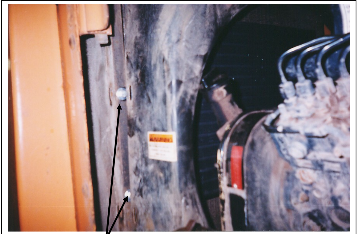
Bolts holding condenser brackets in place
